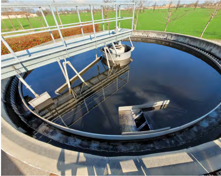
Effluent Treatment Plant in Italy.
